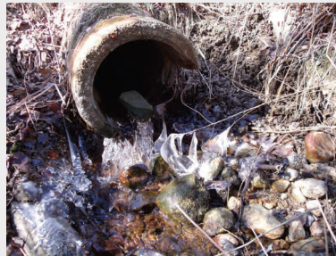
A sub-standard culvert
